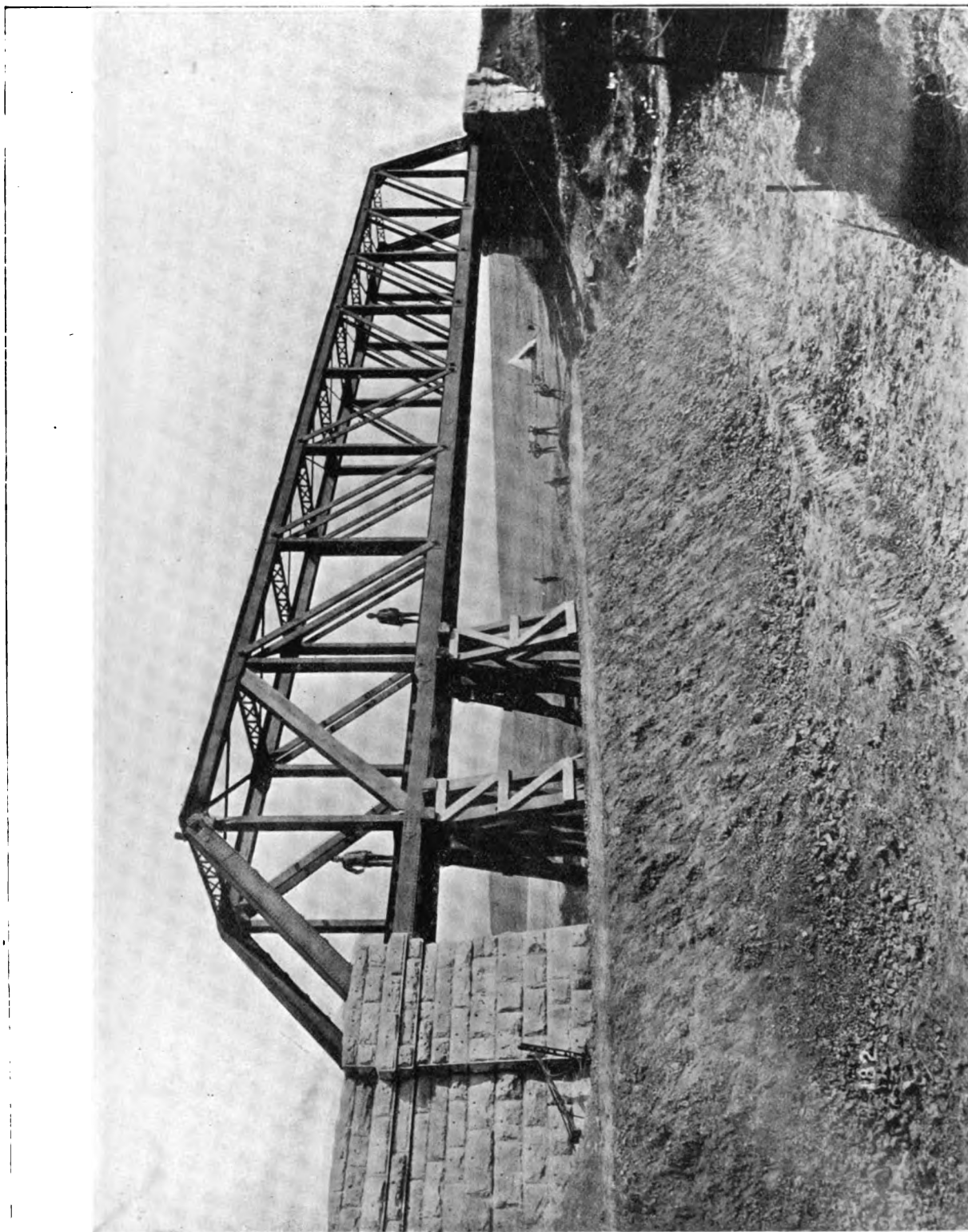
Zandspruit Bridge, Natal. Showing damaged girders supported on trestles.
